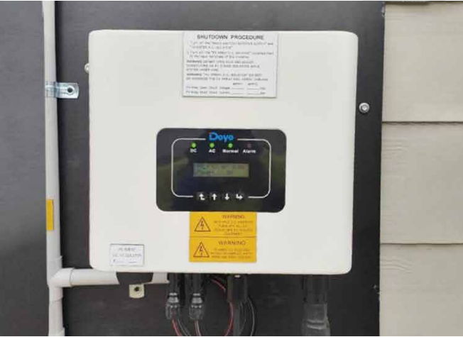
Australia ▶ Inverter: SUN-5K-G Capacity: 5kW
