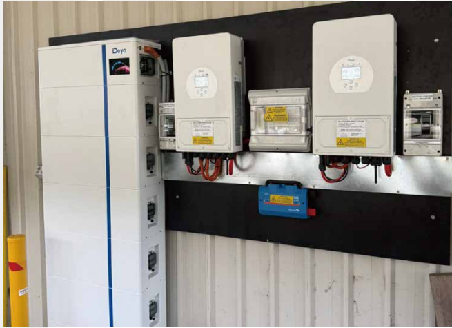
Australia ▶ Inverter: SUN-8K-SG05LP1-AU Battery: AI-W5.1-B-ESS Capacity: 16kW/ 30kWh
