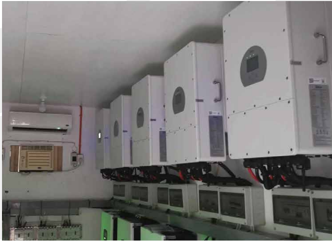
Philippines ▶ Inverter: SUN-12K-SG Capacity: 120kW
