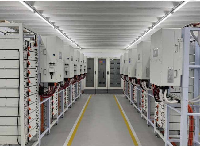
Zimbabwe ▶ Inverter: SUN-50K-SG01HP3 Battery: BOS-G/BOS-G Pro Capacity: 500kW/500kWh
